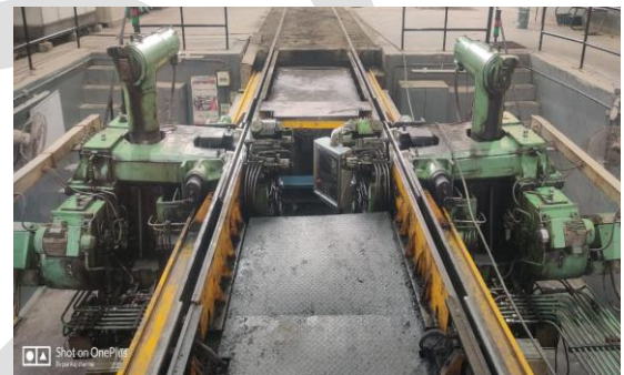
PIT WHEEL LATHE
